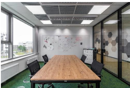
Dynamic Lighting with BIOLUX HCL system in the meeting room
