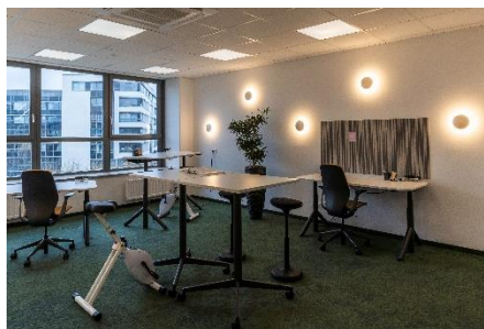
Games Room with VIVARES DALI System und SMART+ wall luminaires
