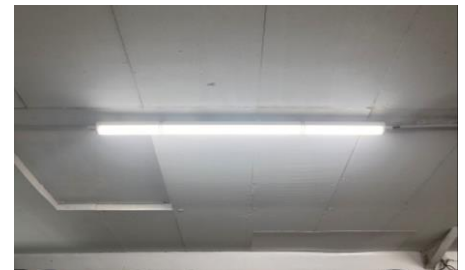
The installation of the DAMP PROOF SPECIAL luminaires was easily implemented.
